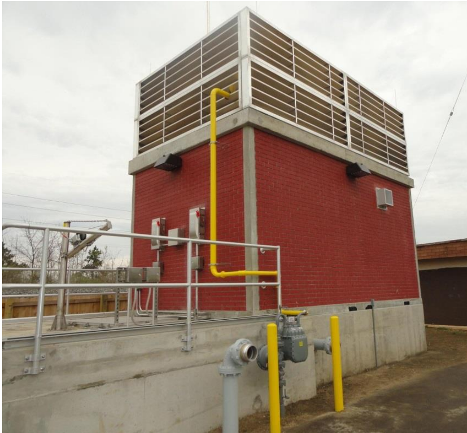
Photo captions: The 77,300 lbs. building was designed for flood conditions up to 5 ft 6 in. and includes a flood-proof water tight door. It supports a roof-mounted 4,100-lb generator.
