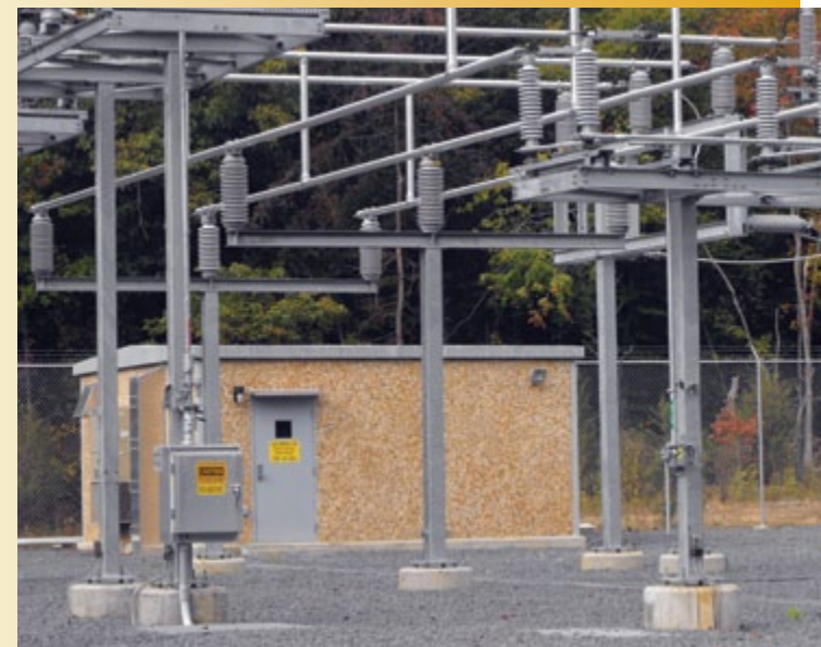
Electrical Sub-Station: Nevada
