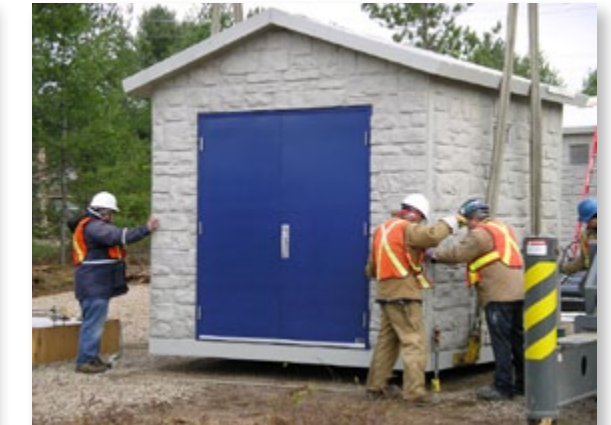
Equipment Building: Ontario, Canada
