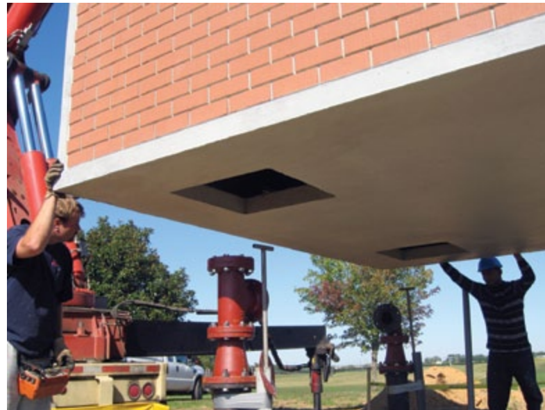
Buildings can easily accommodate existing equipment
