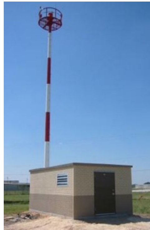
Communications Equipment Housing: Texas
