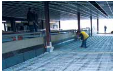
Top-slab, parking garage, Berlin (DE) Thin top-slab for load distribution, shallow concrete cover, corrosion resistant reinforcement. Owner: Forum Steglitz KG, Berlin Installation: 2006
