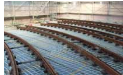
Light rail depot, Basel (CH) Non-metallic reinforcement in floor slab. Owner: BVB Installation: 2009
