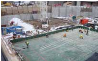
Quantum Nano Center (CDN) Non-metallic reinforcement in foundation slab; undisturbed operation of research equipment. Owner: University of Waterloo Installation: 2008
