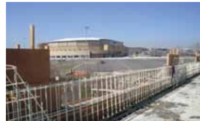
McHugh Street Bridge (CDN) Corrosion resistant highly durable reinforcement in barrier walls. Owner: City of Windsor Installation: 2009
