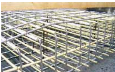
Foundation Slab Transformer Station, Hamneset (NOR) Electromagnetic separation of the foundation from the transformer. Owner: Statnett, Norway Installation: 2006
