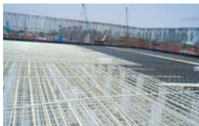
Floor slab aluminium smelter (Qatar) Floor slab in area of rectifiers with nonmetallic reinforcement. Owner: Qatar Petroleum, Norske Hydro Installation: 2008
