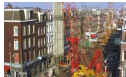
North-South Line Subway, Amsterdam (NL) 80 tons Schöck ComBAR® in the shaft walls for the penetration by the TBM. Owner: City of Amsterdam Installation: 2004 to 2006
